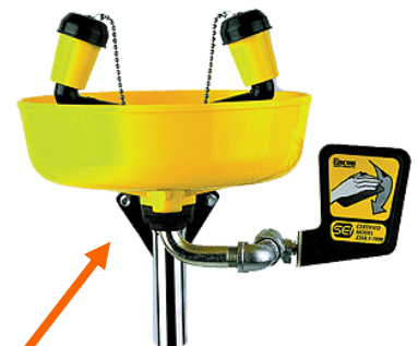
Plumbed eyewash station
