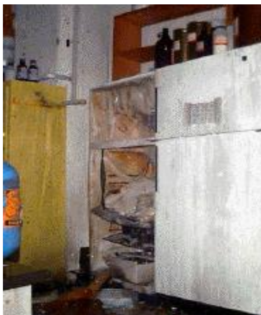
Thermostat inside, left side, caused spark.
